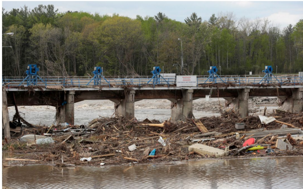
The failed Sanford Dam last week, which flooded the Tittabawassee River and parts of Sanford, Mich. Rebecca Cook/Reuters
