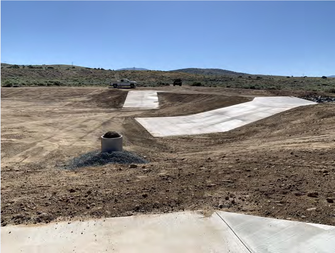
Image showing the inside of one of four flood control basins in the Johnson Lane area in Gardnerville, Nevada. Construction of the basins was completed by Douglas County in August 2023.
